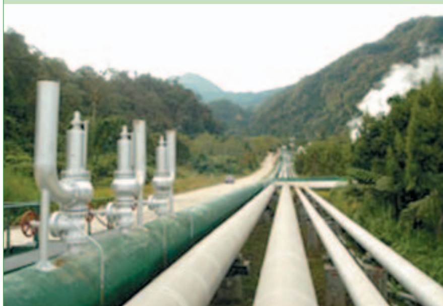
PNOC-EDC is the largest producer of geothermal energy, supplying 12 power plants
